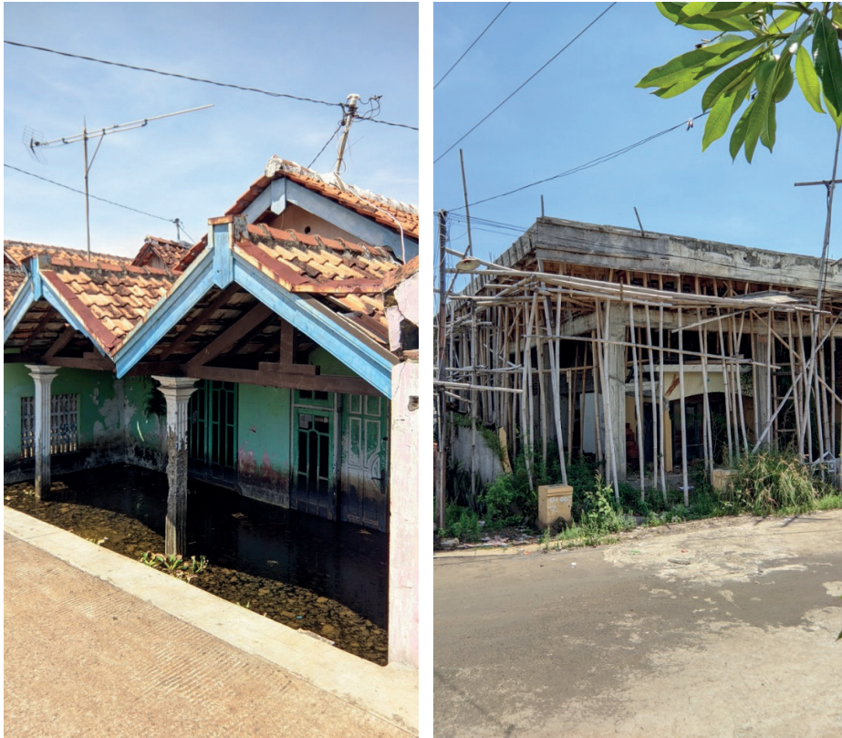
Figure 3-1 Abandoned Property and Structural Adaptation for Distressed Properties
